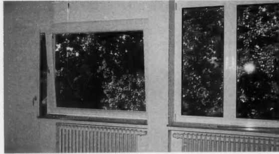
window and door units. On the third floor, these have been replaced by new aluminum-
